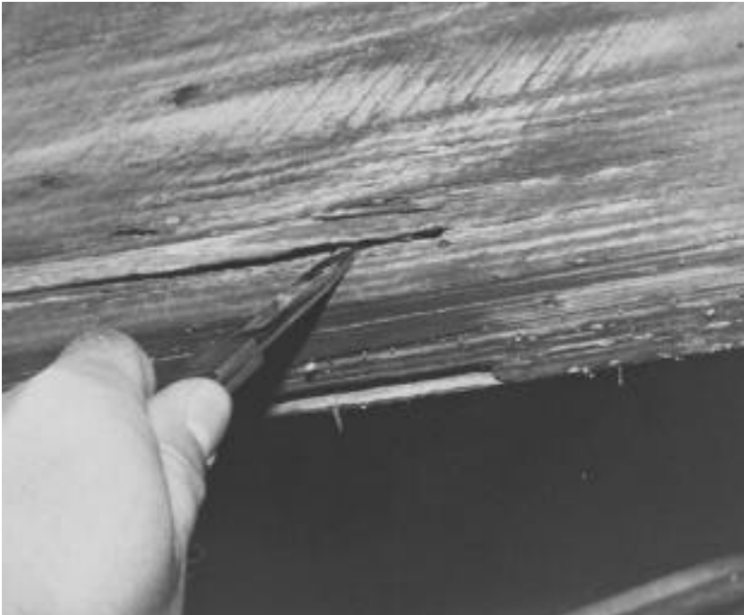
Termite infestation is most common in basements and crawl spaces, particularly near foundation walls. Probe all suspect areas thoroughly.
