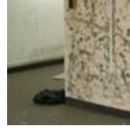
Mold on gypsum wallboard. (photo courtesy of Terry Brennan)
