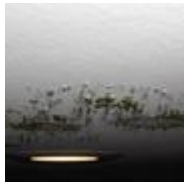
Mold on ceiling. (photo courtesy of Terry Brennan)
