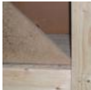
Mold on basement ceiling resulting from chronic high humidity (>90% relative humidity [RH]). (photo courtesy of Terry Brennan)
