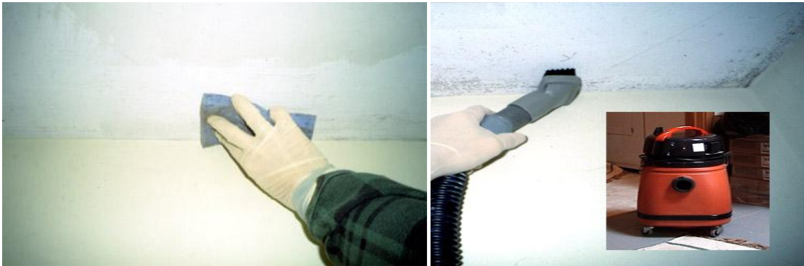
Damp wiping surfaces with water and a small amount of detergent. (photo courtesy of Terry Brennan)
