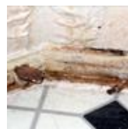
Mushrooms growing at the base of and behind the baseboard below a water leak in a bathroom. The baseboard has been removed; the puckers in the paint are due to water damage. (photo courtesy of John Martyny, Ph.D.)
