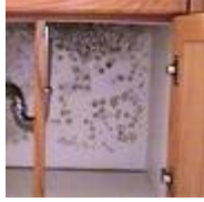
Mold inside a bathroom cabinet where condensation forms. (photo courtesy of Terry Brennan)
