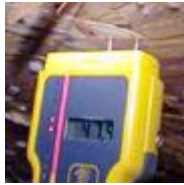
Moisture meter and moldy roof sheathing. (photo courtesy of Terry Brennan)
