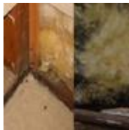
Looking for mold in wall cavities by removing a section of drywall. (photo, John Martyny, Ph.D.)
