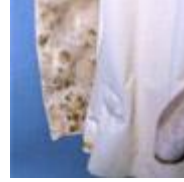
Mold on shower curtain. (photo courtesy of Terry Brennan)
