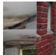
Mold on first floor beneath a through-the-wall air conditioner on the second floor. (photo courtesy of Terry Brennan)
