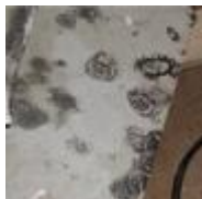
Sections of moldy gypsum board. (photo courtesy of Terry Brennan)
