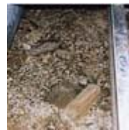
Mineral deposits on the surface of a dirt crawl space caused by chronic water problems. (This is not mold.) (photo courtesy of John Martyny, Ph.D.)
