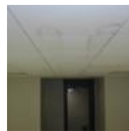
Water-damaged ceiling tiles. Air conditioning ducts above the ceiling were not insulated in several areas resulting in condensation on the ducts that dripped onto the ceiling tiles. (photo courtesy of Terry Brennan)
