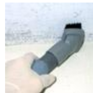
HEPA vacuum. Care is being taken to disturb the mold as little as possible while vacuuming. (photo courtesy of Terry Brennan)
