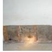
Mold inside a wall. This photo shows an interior wall with the lower portion of the drywall removed on one side; there is mold on the backside of the drywall caused by water leak. (photo courtesy of John Martyny, Ph.D.)
