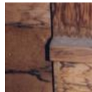
Wood showing water stains caused by roof leak.
