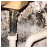
Mold on drywall under leaky sink. (photo courtesy of John Martyny, Ph.D.)
