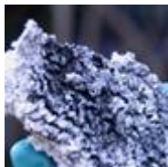
Mold on fragment of ceiling tile.
