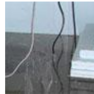
Several inches of water in a basement with a broken sump pump. (photo courtesy of Terry Brennan)
