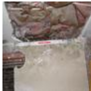
Opening a wall with a utility knife to minimize disturbance to mold in the wall cavity.
