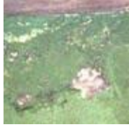
Water from roof leak has seeped into a wall causing the paint to buckle and peel. (photo courtesy of Terry Brennan)
