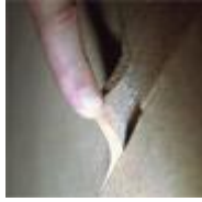
Most mold is found by simply looking. Mold beneath corkboard. (photo courtesy of Terry Brennan)
