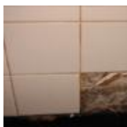
Mold growth under ceramic tiles in a bathroom. (photo courtesy of John Martyny, Ph.D.)
