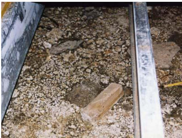
Mineral deposits on the surface of a dirt crawl space caused by chronic water problems. (This is not mold.) (photo courtesy of John Martyny, Ph.D.)
