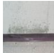
Mold on painted concrete in a school building. Rainwater is wicking directly through the concrete walls, and there is also condensation on the earth-chilled concrete. (The floor is about 3 feet below ground level.) (photo courtesy of Terry Brennan)
