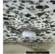
Extensive mold contamination of ceiling and walls. (photo courtesy of Terry Brennan)
