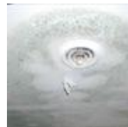
Mold surrounding air conditioning vent in ceiling due to water leak. (photo courtesy of John Martyny, Ph.D.)
