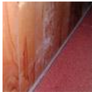
Mold on wooden paneling. (photo courtesy of Terry Brennan)
