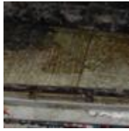
Mold (and dirt) beneath refrigerator due to chronic drip-pan overflows. (photo courtesy of Terry Brennan)
