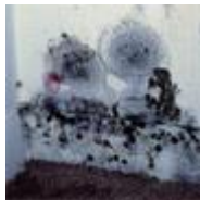
Moldy bedroom closet. Water condensed from the air onto the gypsum board. The wall is cool enough for condensation because there is a hole in the insulation and it is cold outdoors. (photo courtesy of Terry Brennan)
