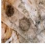
Mold growing on oriented strand board used for structural wood floor in crawl space. (photo courtesy of John Martyny, Ph.D.)
