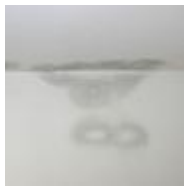
Water stains on wall and ceiling. (photo courtesy of John Martyny, Ph.D.)
