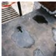
Puddles on flat roof.
