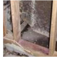
Mold inside a wall cavity. (photo courtesy of Terry Brennan)
