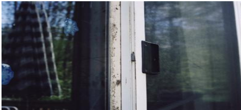
Mold on the air seal of a sliding glass door.
