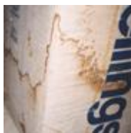
Water stains in basement. (photo courtesy of Terry Brennan)
