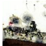
Colorful mold growth. (photo courtesy of Terry Brennan)
