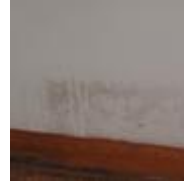
Basement apartment (3–4 feet below ground) with mold on painted gypsum board, baseboard, and carpet. (photo courtesy of Terry Brennan)
