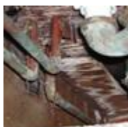
Moisture damage and mold growth under bathtubs. (photo courtesy of Terry Brennan)
