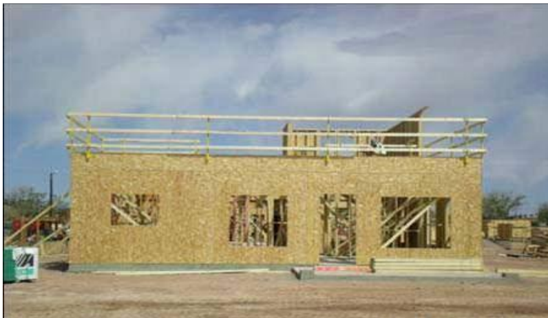
Here is a 2nd floor perimeter completely protected by a guard rail system.
