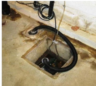
Sump hole – clear cover-sealed
