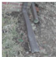
Moisture issue: Foundation is wet; drain gutters are too short. Fix: Drain rain water away from the house, generally about 5 feet away from the foundation. Gutters below grade (below the soil) are protected from damage, while those above grade may be more easily damaged.
