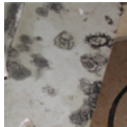
Sections of moldy gypsum board.
