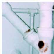
Rust is an indication that condensation occurs on this drainpipe. The pipe should be insulated to prevent condensation.
