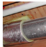
Moisture issue: Condensation on uninsulated air conditioning duct. Fix: Insulate the duct on the outside. (photo courtesy of Terry Brennan)
