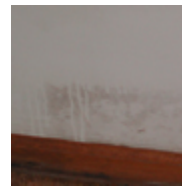
Basement apartment (3-4 feet below ground) with mold on painted gypsum board, baseboard, and carpet. (photo courtesy of Terry Brennan)
