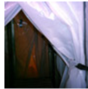
Full containment. (photo courtesy of Terry Brennan)
