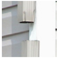
Moisture issue: Disconnected downspout deposits rainwater from roof onto walls and near foundation. Fix: Connect the 2 downspouts. (photo courtesy of Terry Brennan)
