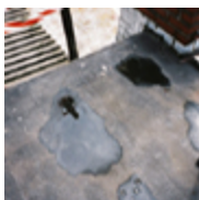
Puddles on flat roof.
