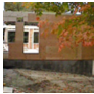
Moisture Issue: Foundation was chronically wet, water and mold damage was found on original structure. Fix: Area was regraded during construction of an addition so that water drains away from the foundation.
